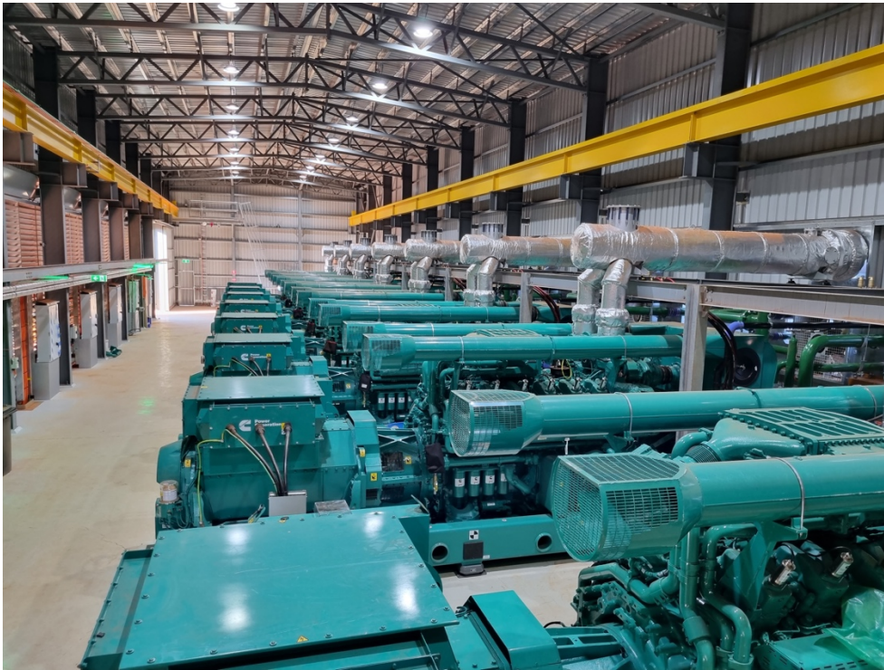
Inside the engine hall
